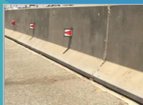
Dome Concrete Barrier Reflectors
